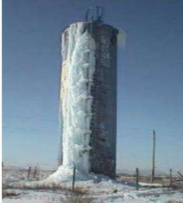
Frozen finished water storage tanks
