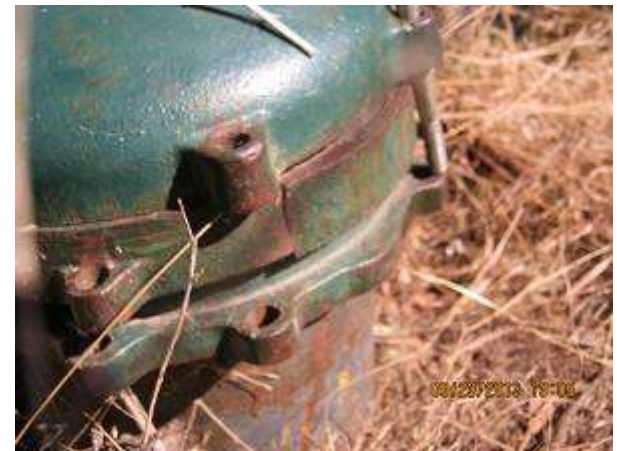
Lack of bolts creates the lack of a sanitary seal
