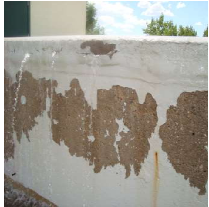
Leaking finished water storage tanks
