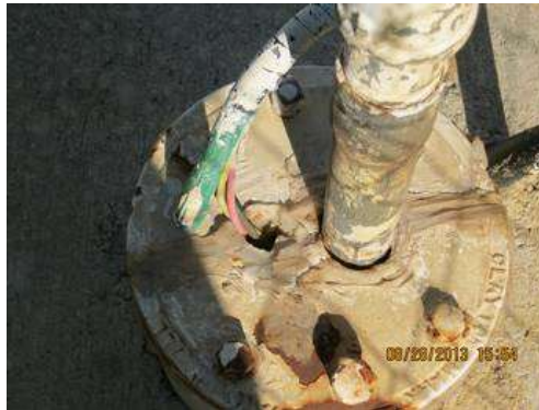
Lack of a sanitary seal and proper well cap
