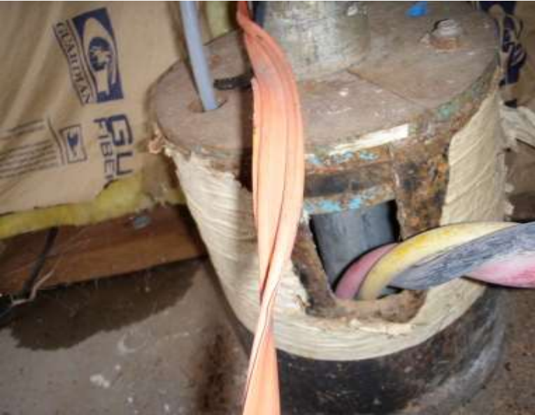
Conduit is not properly sealed
