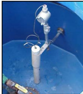
Float sump sensor
