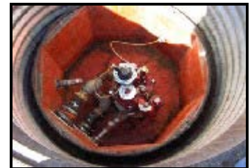
Contained turbine sump
