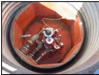
Dry, debris-free contained turbine sump
