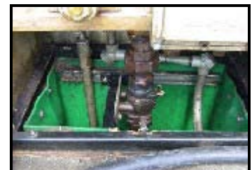
Contained dispenser sump
