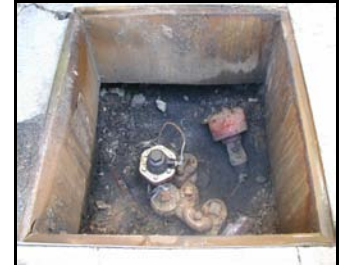
Uncontained turbine sump
