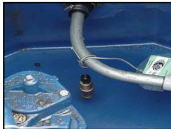
Liquid sump sensor
