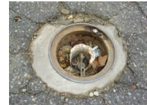
Monitoring well with missing cover and filled with debris
