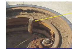
Tank top sump sensor installed too high
