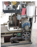
Suction piping system
