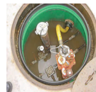
Tank top sump full of liquid
