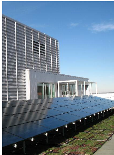
Solar panels on a green roof
