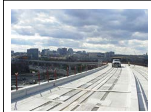
Exhibit B-4. Construction of the Metrorail extension in Fairfax County, Virginia. Source: Stephen Barna via Flickr.com.
