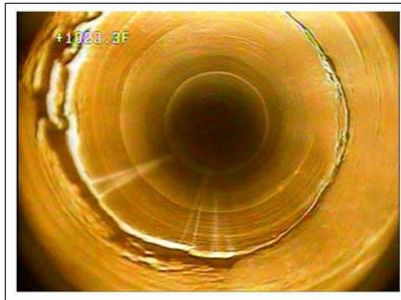
Figure 6. Video still image of saline-water inflow from a bedding-parallel fracture penetrated at 1,026 feet below land surface by the Gleason corehole, western Bradford County, Pennsylvania
