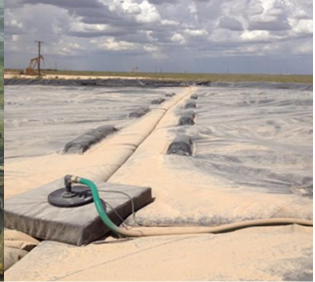
Figure 4. Pond Cover over freshwater storage
